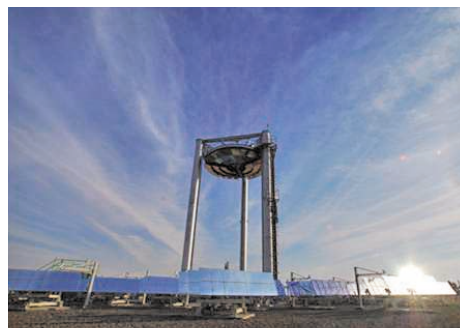
CSP generation demonstration plant
